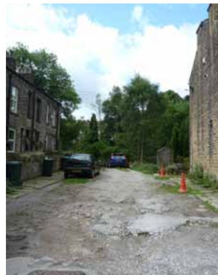
Poorly maintained road surfaces
