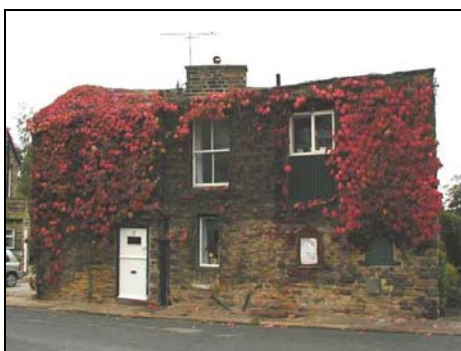
2 Victoria Street (key unlisted building). The partially blocked loading door is above the notice board to the right.
