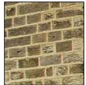
Regularly coursed stone 'brick' with an unobtrusive lime-based mortar at Peas Acre.
