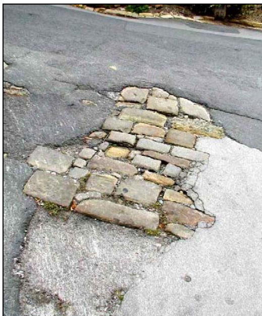
Patched up road surface near High Fold.
