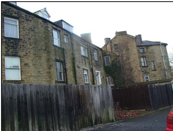
Rear of the properties from Sir Wilfred Place – the image could be enhanced by the better detailing of stone wall boundaries.
