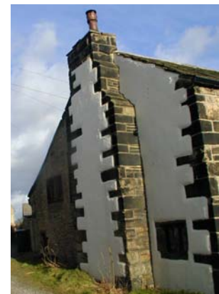
Large stone chimney stack of 30 Westfield Lane (Grade II) – Late 18 th century cottage.
