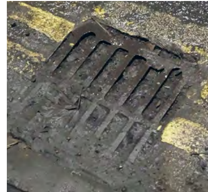
adequately maintain existing drains
